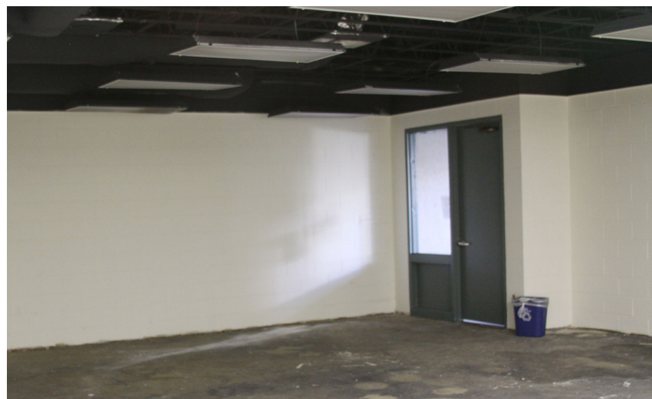
The Ludd M. Spivey Fine Arts Center undergoes construction as the English department moves out.
